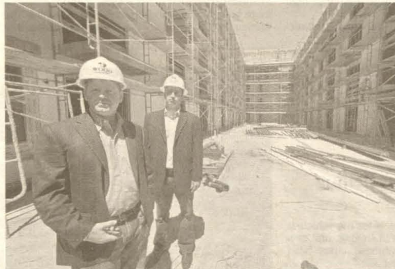
Work has resumed at City Walk, above, after three years. Frank Middleton, left, and Brian Pianca of Wood Partners, which is finishing the project.
